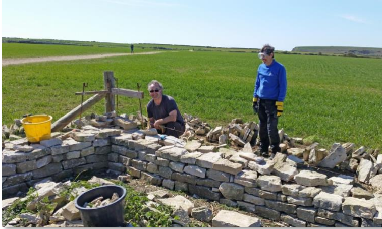
Saturday - Ian and Tim work on building the corner of the wall ...
