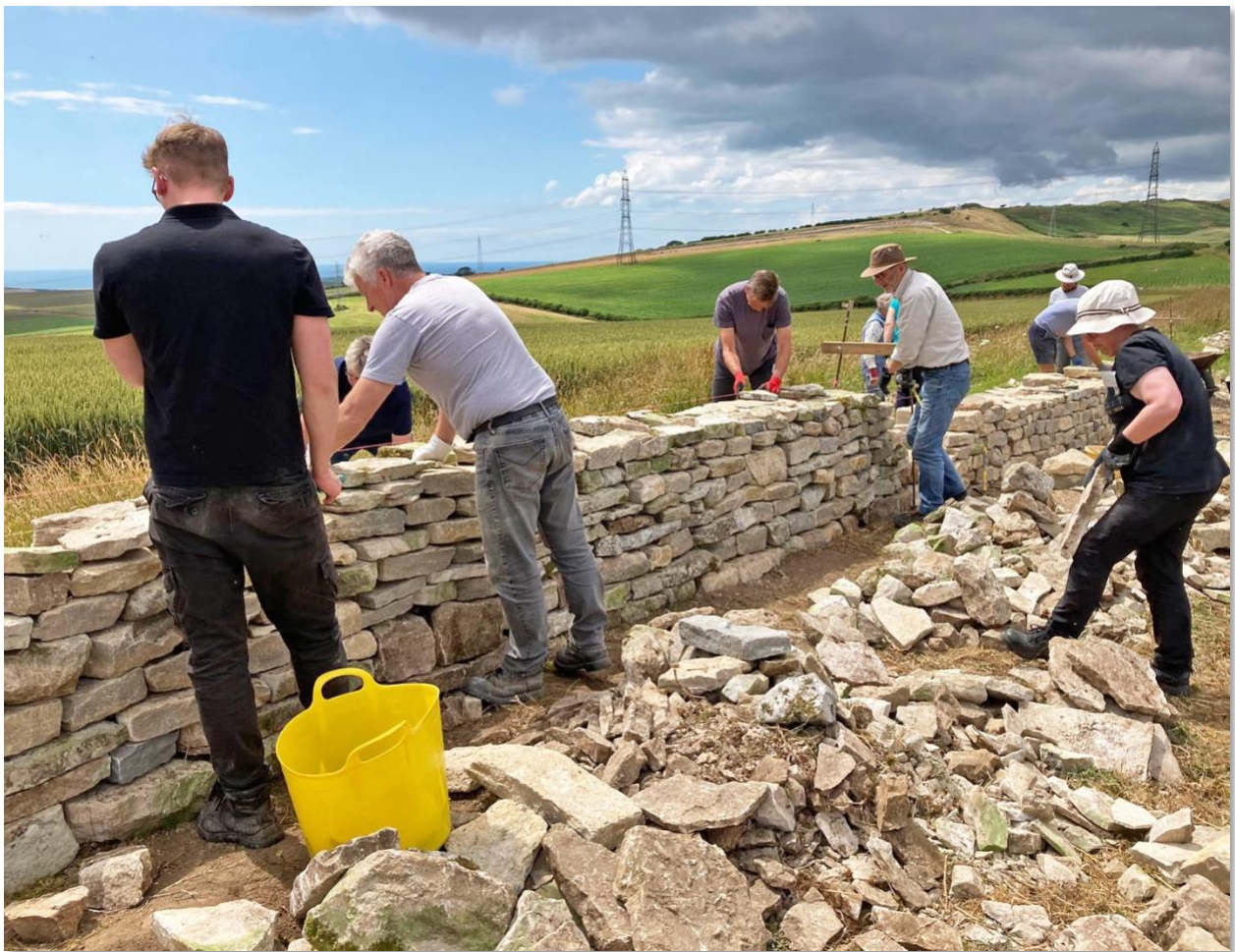
Day two and second lift. These wallers are fast learners and seem to have an affinity for the stone. But of course, they are being well taught!
