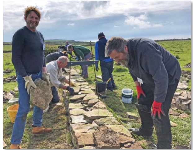
Left: Peter's group making a nice job of straight coursing – difficult here because the wall is on sloping land. In fact, this isn't an easy site for a novice wall although it is one of the most peaceful and stunning locations on South Purbeck.
