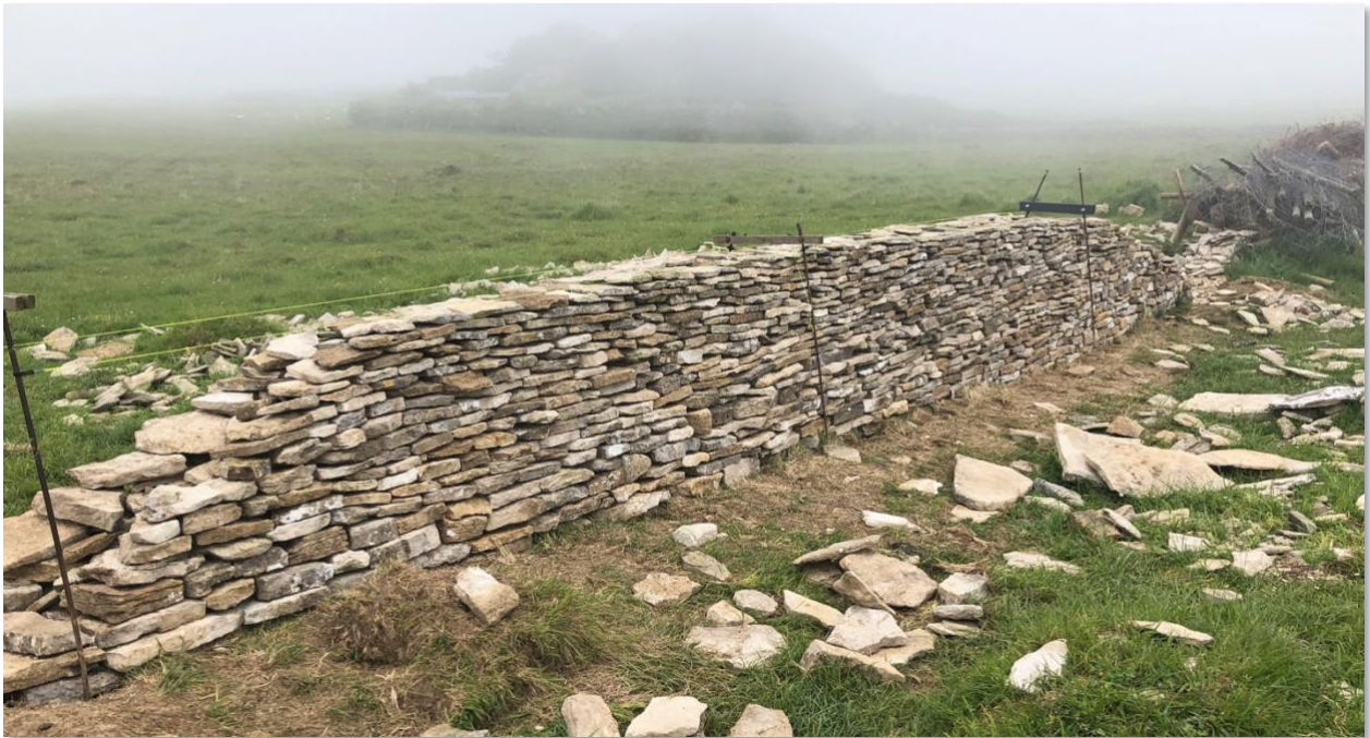
On Sunday, I am on my own so I'm not able to complete the wall and cope it. Nevertheless, I get a good section to height and repair the sheepwrecked wall as far as possible. Now that we have some heavy foundation stones, we'll be able to begin dismantling and rebuilding the entire wall. However, as you can see in this photograph there is a huge pile of old barbed wire fencing to be removed before we can go much further.
