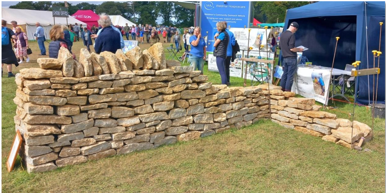
The finished wall looks great, especially with the corner as an additional feature.
