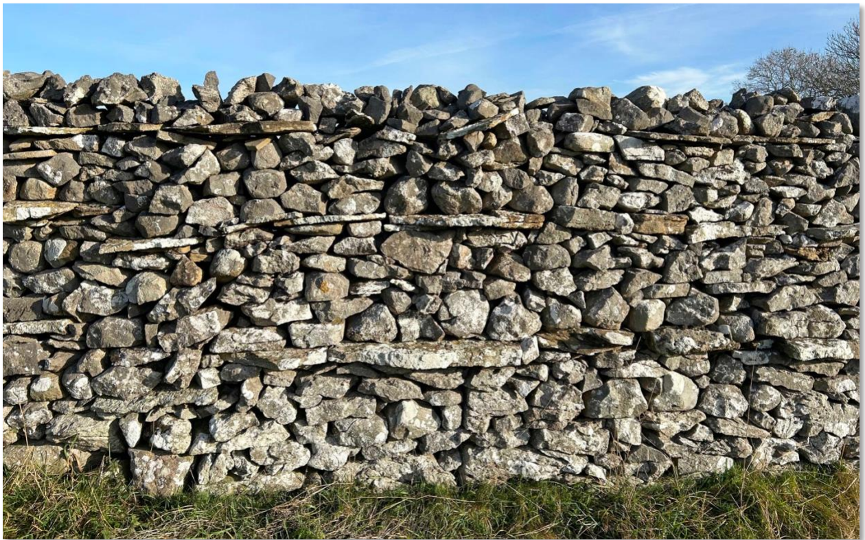
Harder than it looks to create a wall like this. Note the typical Yorkshire through stones sticking proud of the wall.
